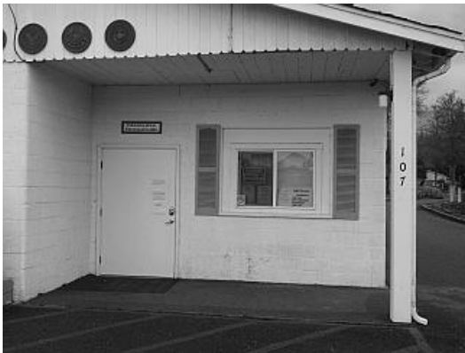
Photo of entryway at Post 62 showing the new vertical support beam that was installed on March 17, 2020. The new beam has our street address number 107. The rain gutter downspout on the beam was also replaced. The building's roof was treated to retard moss growth.
