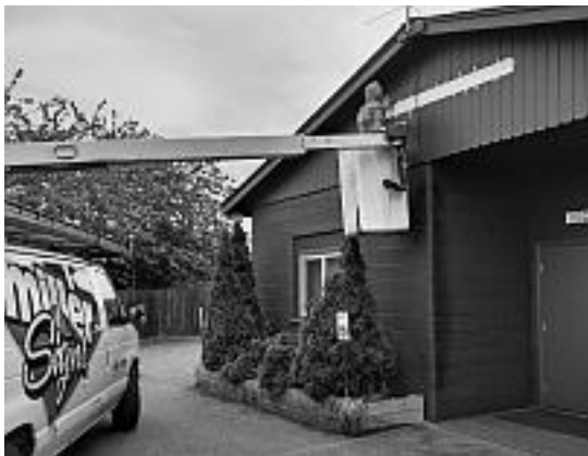
This is a photo taken at Post 62 on May 25, 2024. This shows the new "American Legion, Jack Grennan, Post 62" sign on the front of our building being installed.
